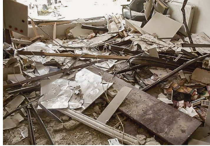
A collapsed ceiling in the center for the elderly; now the home is being rebuilt. csi
